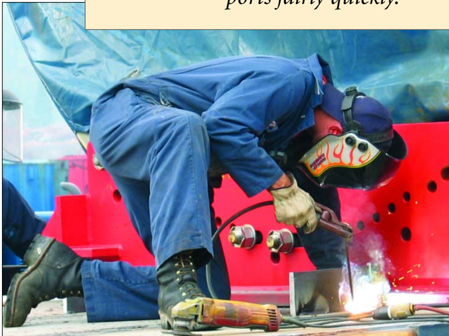
Welding and other services are sometimes needed to accommodate the needs of cargo shippers. Photo courtesy of the Port of Longview.
